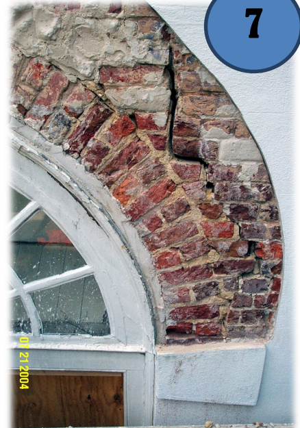
Brick under stucco, 2004 repairs on the west wall; courtesy of Richard Marks Restorations and Old St. Andrew's.
